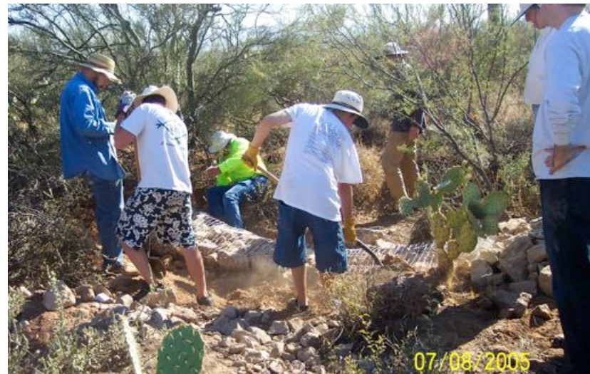
Above: Scenic Drive Watershed Restoration Project in conjunction with the town of Marana and SaPWET, installing a gabion. July 2005.
