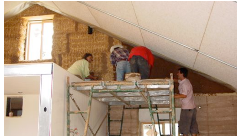
Above: Strawbale gable walls being plastered with onsite clay and plant fibers
