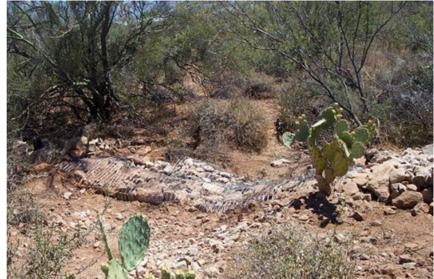
Gabion after summer 2006 rains.
