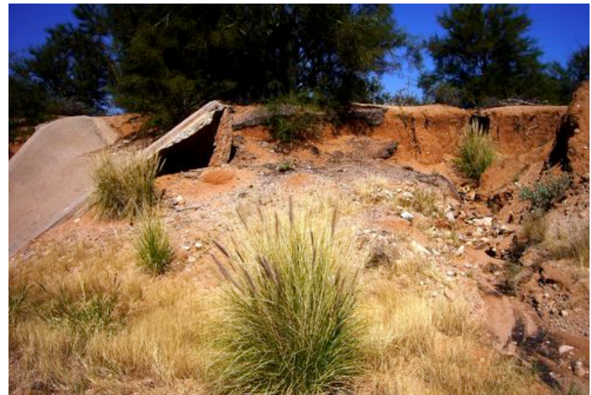
Erosion cuts a new channel perpendicular to concrete drainage structure.
